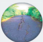
Surface Distress / Cracking
